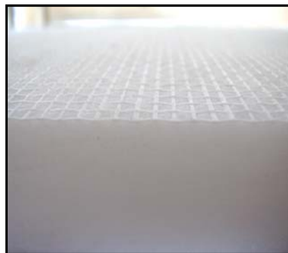
Paint Booth Intake
